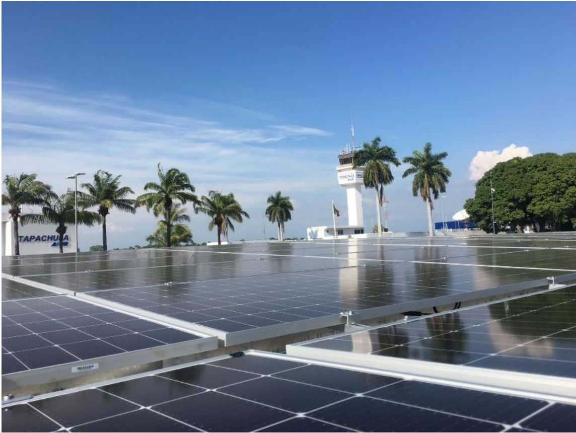
Image 2. Solar panels at Tapachula Airport
