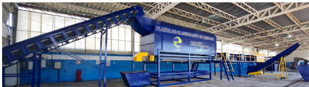
The waste separation plant at Cancun Airport with the project's new investments
